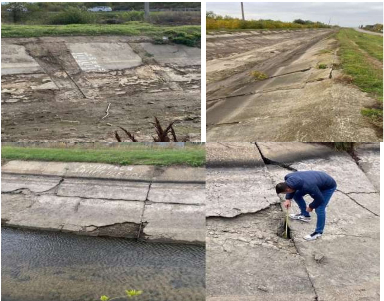
Figure 1. Damage to the anti-filtration coating of the main channel of the 1st stage of the Engels irrigation system
